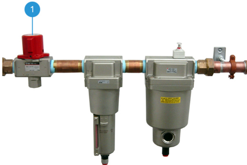
Figure 1. Compressed air supply shutoff valve and canisters
